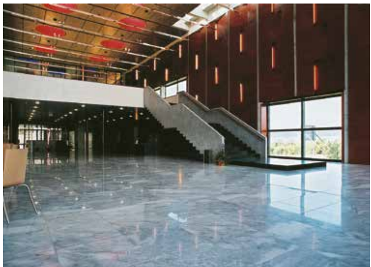
An example of the installation of a marble floor - Feuchtwangen casinò hall (Germany)
